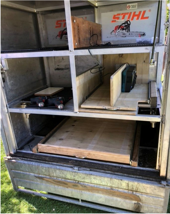
Fig 6: Sliding trays for the chargers were installed in the rear section of the trailer.
