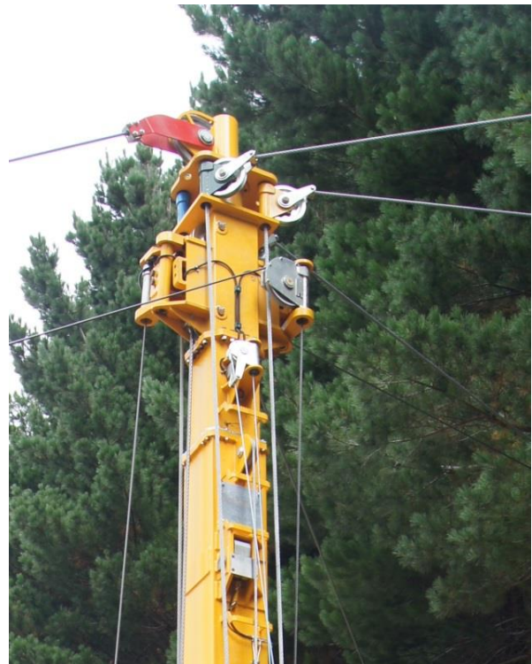
Figure 5: Top of the Koller tower showing rope guides on the guyline and skyline sheaves.
