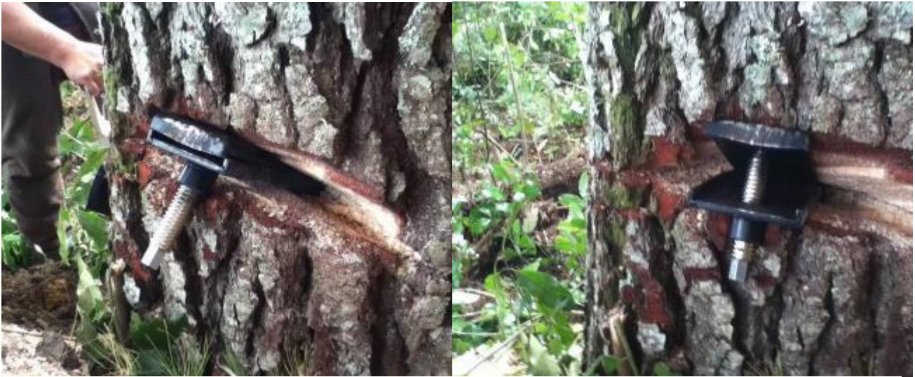
Figure 7: Sloping back cut (left) and enlarged back cut (right) trialled for effectiveness
