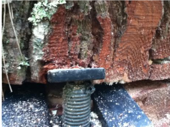
Figures 16: JBL wedge in tree with fluting removed to accommodate the screw pin
