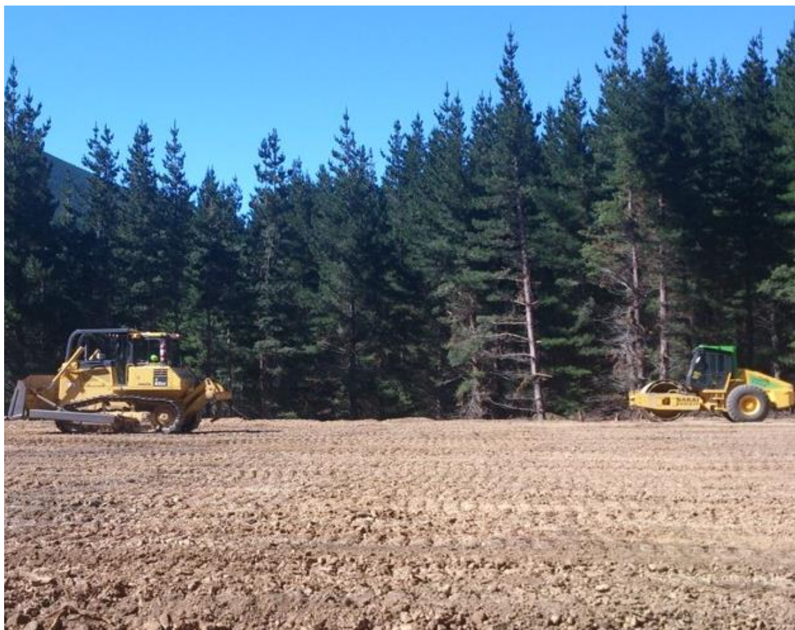
Figure 2. Summertime landing construction in Canterbury. Compaction involved track-rolling the landing with a Komatsu D65 EX bulldozer (left) prior to vibratory rolling with a Sakai SV512TF (right).
