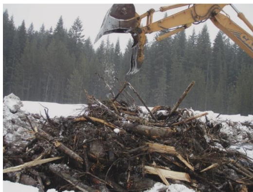
Figure 9. A machine constructing an elevated pile. Source: J. G. Archuleta (PageDumroese et al. , 2017)
